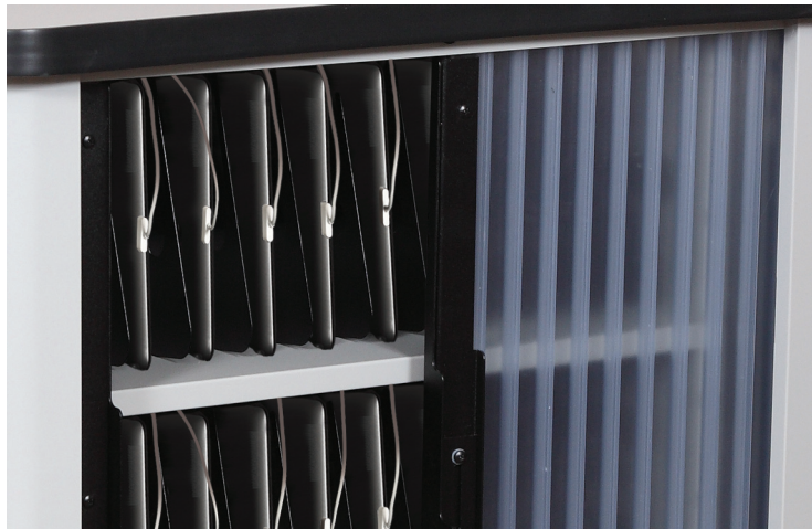
Figure 4-1. Sync cables in cart unplugged from iPads.
