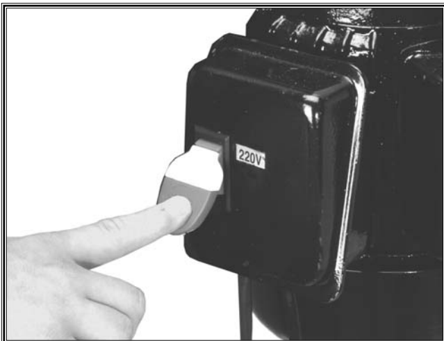
Figure 41. Ready for emergency shut down.
