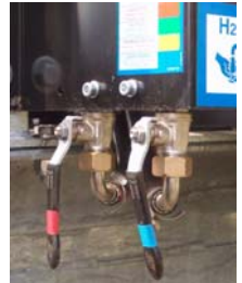
Tank washing tap (BLUE)
