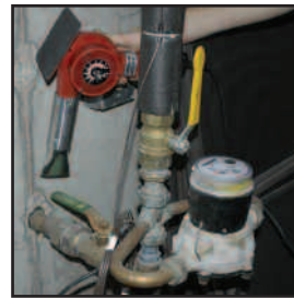
Thaw Frozen Pipes
