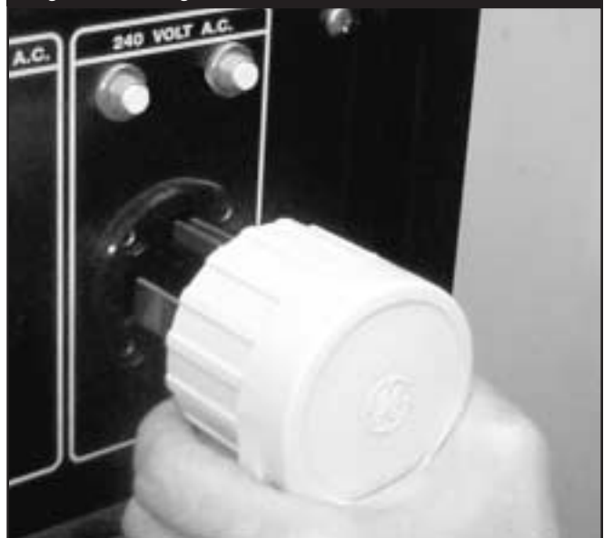
Figure 20 — Align Connector at Generator
