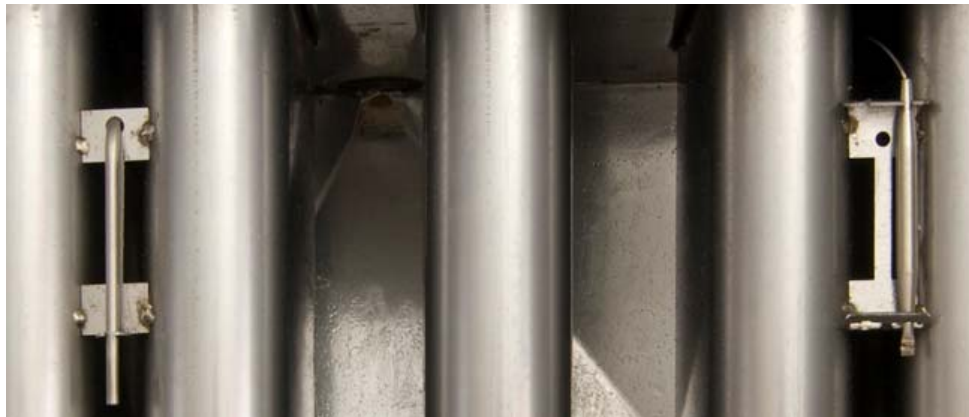
Typical sensor probe/high-limit locations and mounting hardware.
