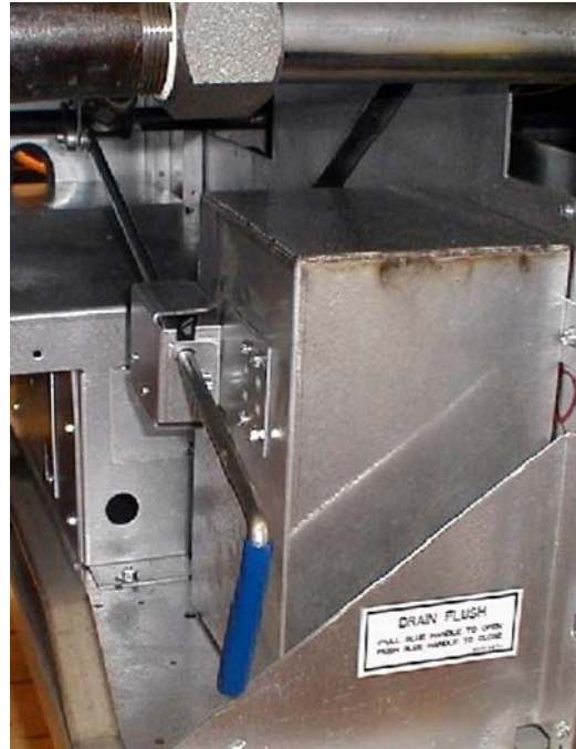
Drain-flush handle (blue) location.
