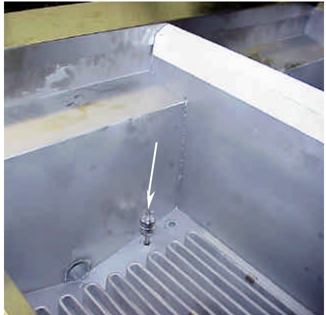
Float safety switch location.
