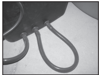
Unused outlets connected with tubing
