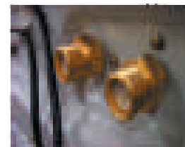
Brass Pressure Regulators installed on back of appliance.
