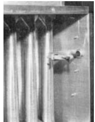
View of limit switch from "inside" the furnace
