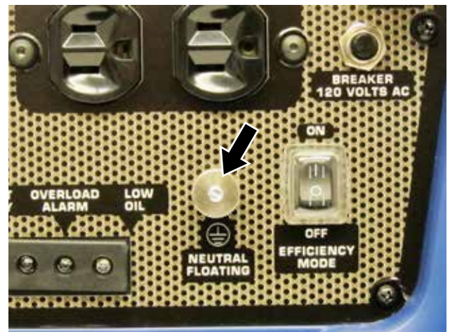
Figure 13 – Ground Terminal on the Control Panel
