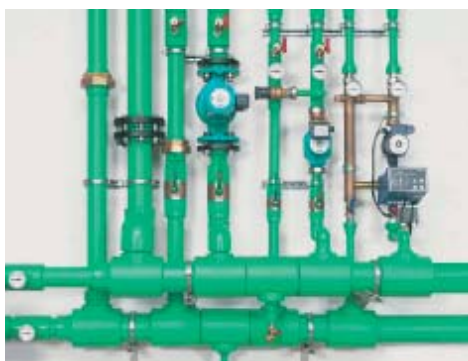
Industriale - Industrial - Industriel
