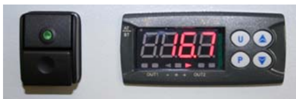
Detail of command panel of refrigeration group.
