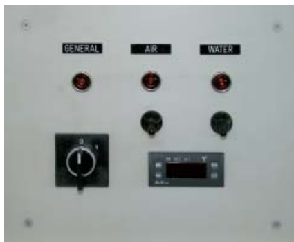
Detail of cabinet control panel.
