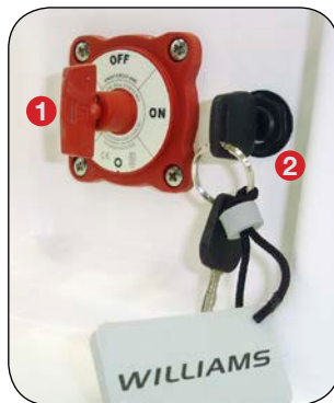
1 Battery isolator switch 2 Key switch
