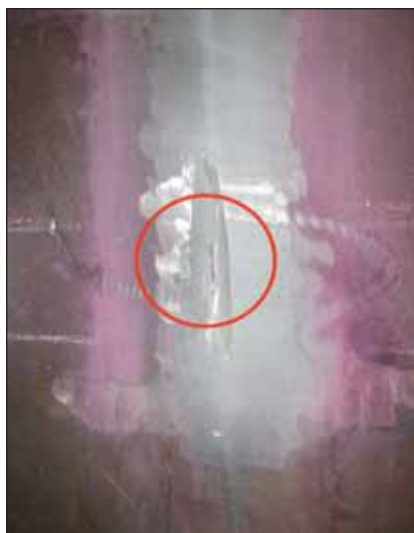
Figure 20 - View of dye penetrant test on defect shown in Figure 19 after excavation.
