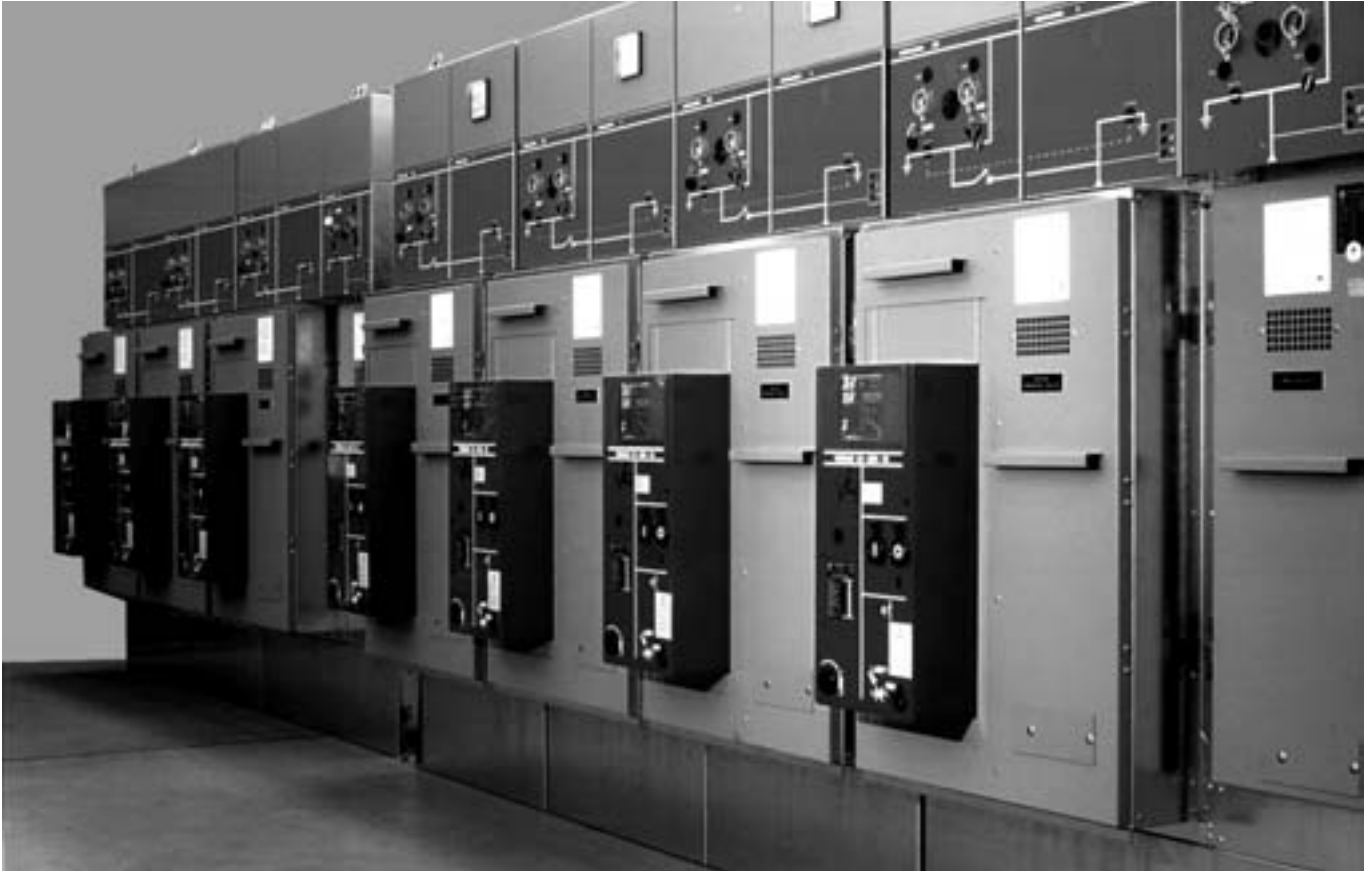
Quadro UNIFLUORC completo di rele' ed interruttori isolati in gas SF 6 (VEIGAS) UNIFLUORC switchboard equipped with relay and circuit breaker insulated with SF 6 gas (VEIGAS)
