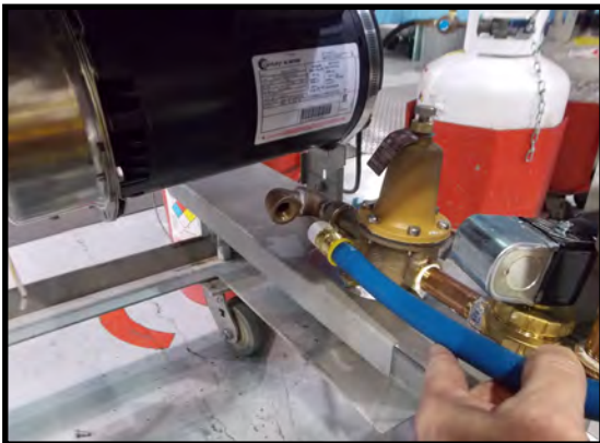
C. PRV Inlet from Coil
