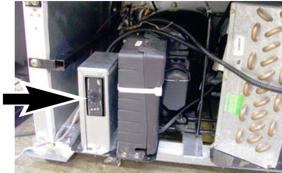
Safe-NET III Controller Location
