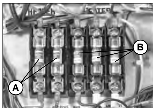
Figure 12 Fuses (Three phase shown)
