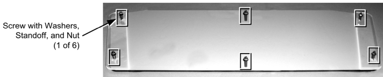
Figure 3. Back of the Marquee Face
