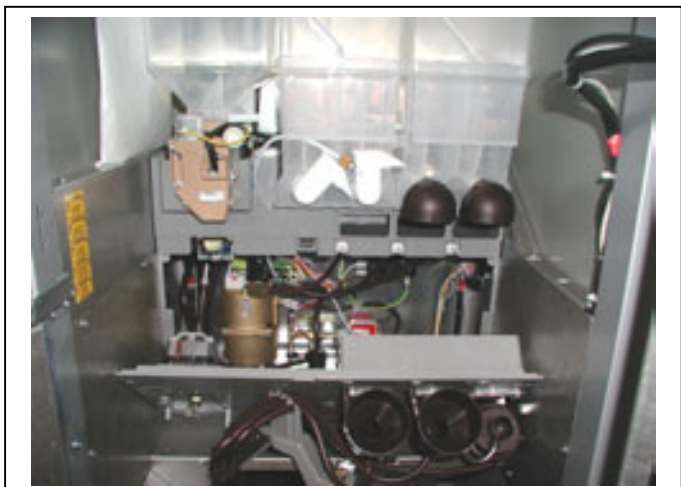
VIEW OF ESPRESSO BOILER COMPARTMENT WITH PUMP (MIXER SUPPORT WALL TILTED)
