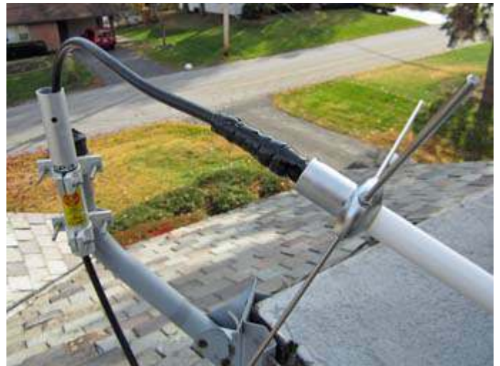
Coaxial cable was connected to the antenna base then wrapped with Scotch 2228 moisture sealing tape and Scotch Super 88 vinyl tape for protection.
