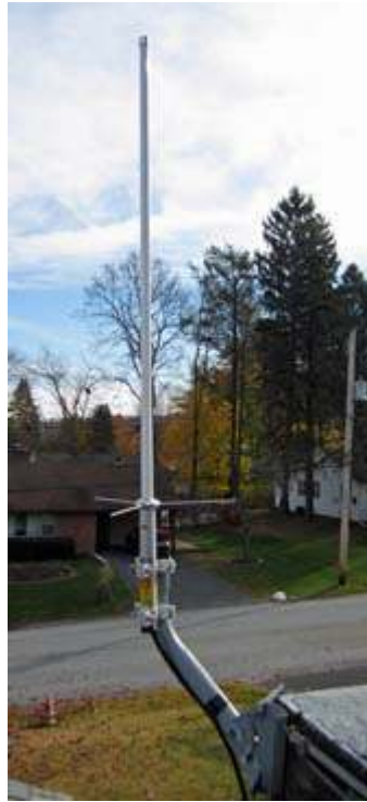
Comet GP-1 antenna in final position, with coaxial feeder taped to the support.
