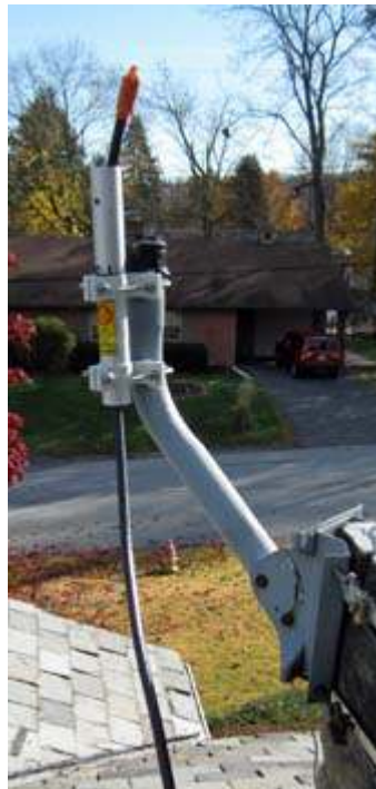
Coaxial cable is passed through the antenna support pipe. (The orange tape protected the PL-259 plug).
