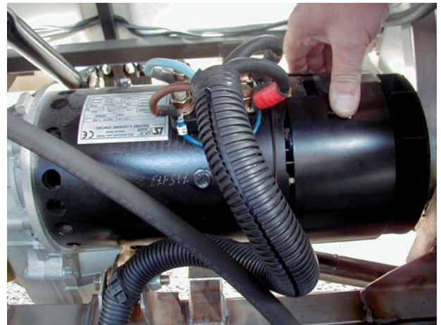
Plate fitted incorrectly (wrong way round)
