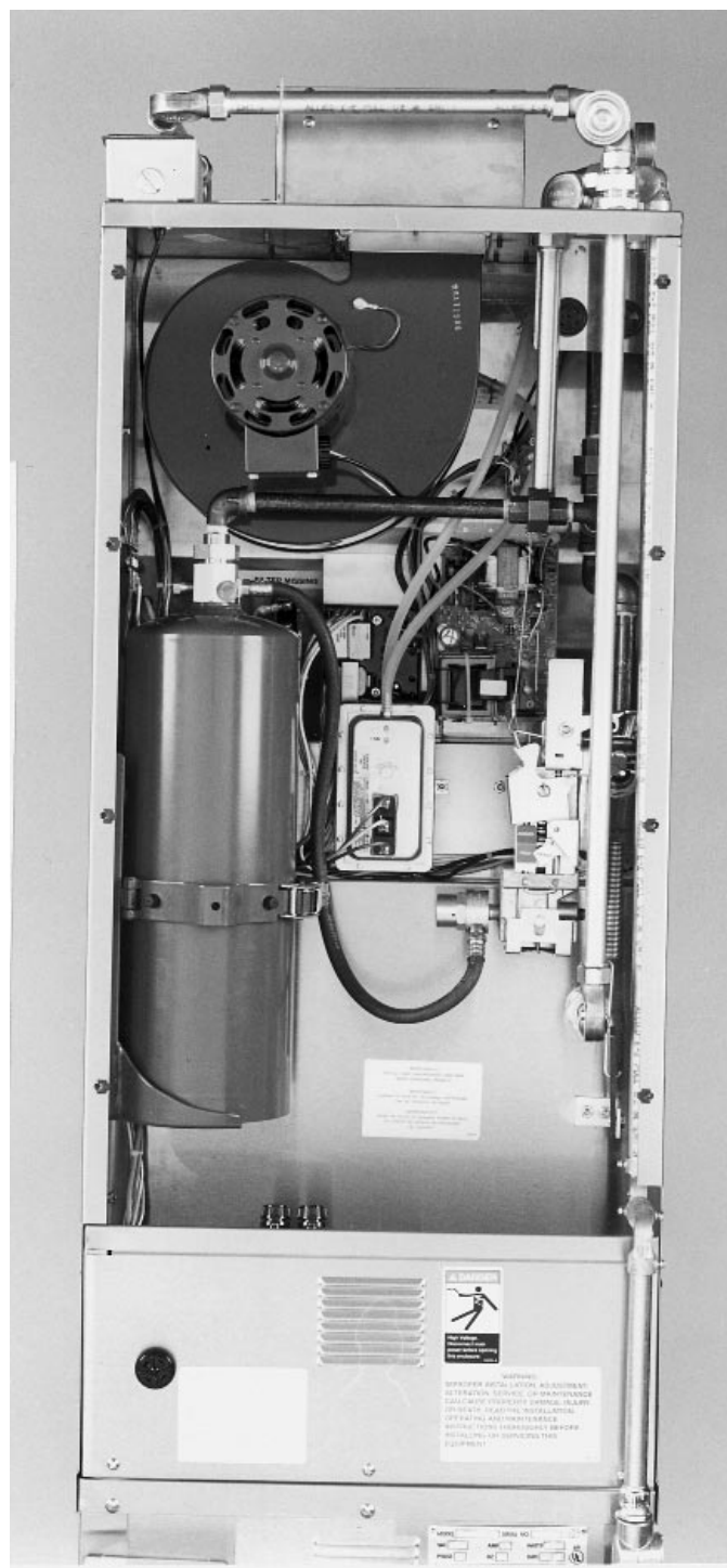
Upper Rear Panel Removed Showing Location of Fire Suppression System Figure 12
