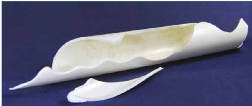
Burst PVC piping from a compressed air installation.
