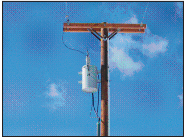
Overhead Power, Pole and Transformer
