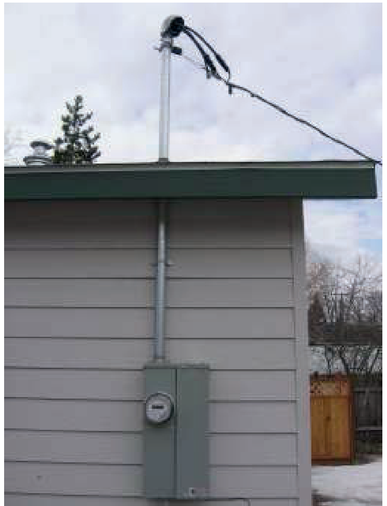
FIGURE 1-11 Surface mounted meter socket
