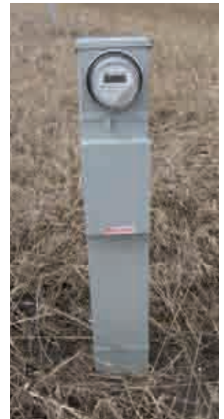
FIGURE 1-17a Factory built meter pedestal
