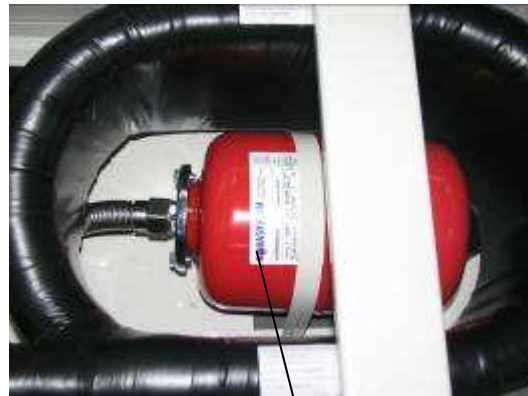
Expansion gas tank
