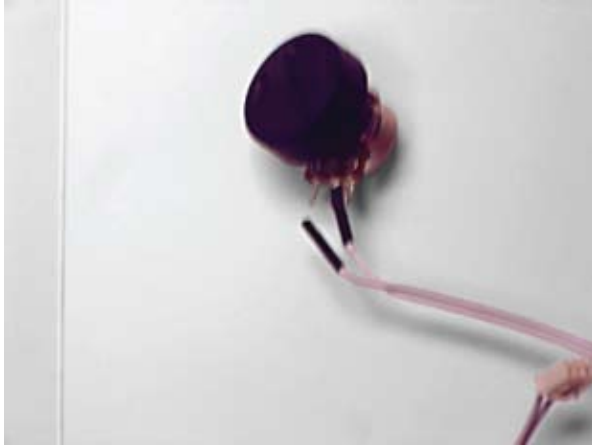
Figure 22, example of bad connection at temperature pot
