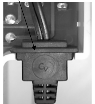
Direct Wire Rack.
