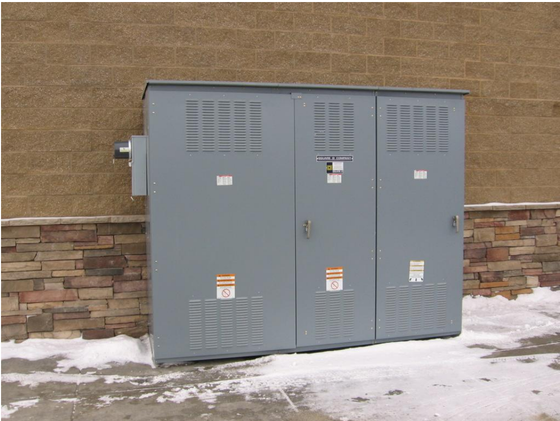
Photo 4: Switchboard metering cabinet with meter base mounted to cabinet.
