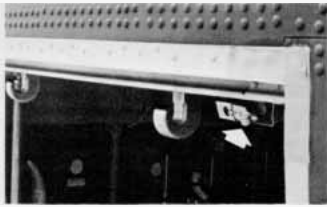
Figure 14. The door closed switch is located near the upper aft corner of the door opening.
