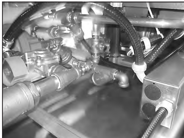
Hot water connection
