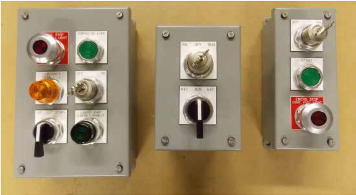
Automatic Cycle with Advance Warning Light and Dumper Remote Control Station
