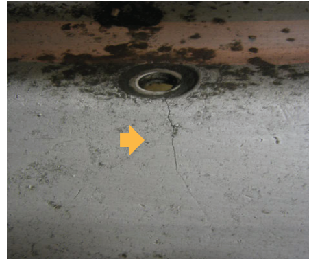
Valve hole crack
