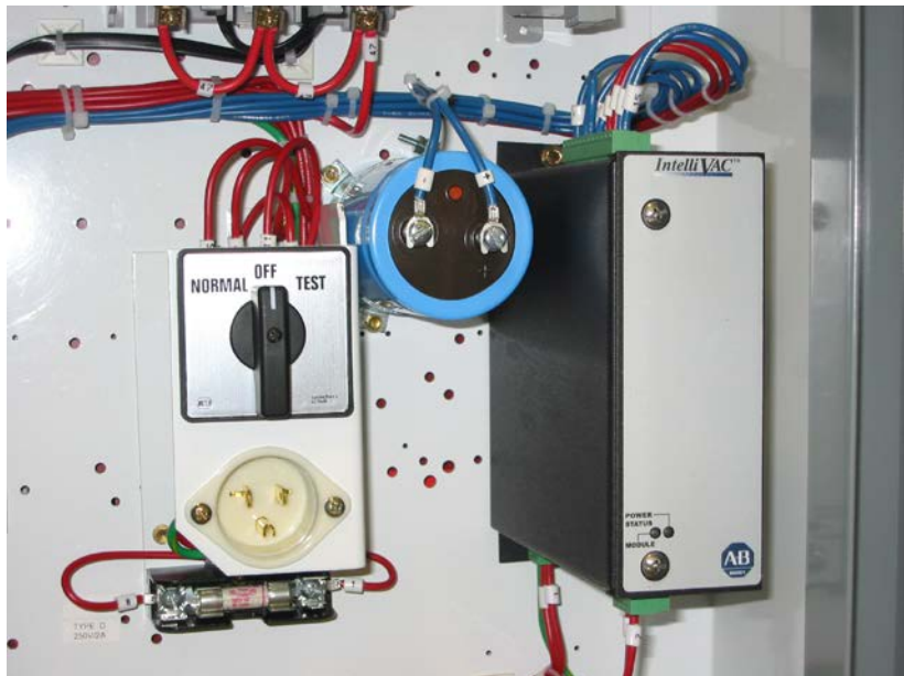
Figure 3.1 – Typical IntelliVAC Installation within a Bulletin 1500/1900 MV Controller (Shown with optional external capacitor)
