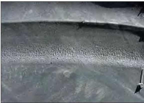
Abrasion marks on the sidewall
