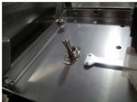
De-lime switch in control box
