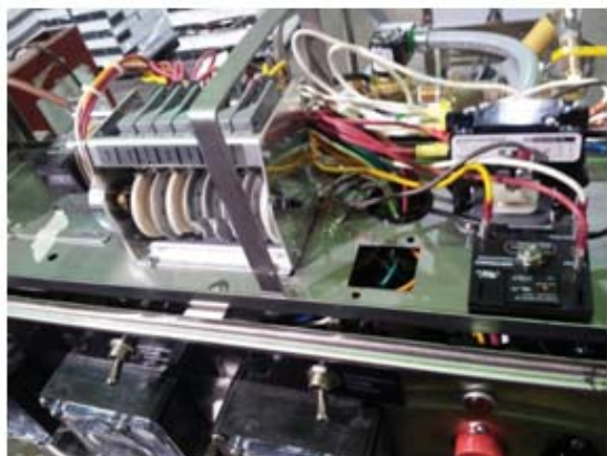
Showing control tray installed in normal position
