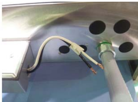
Showing power connection box for 120v wiring
