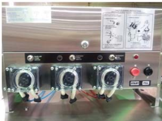
Showing the control box with chemical pumps, prime switches, red start and black fill switch, chemical tubes
