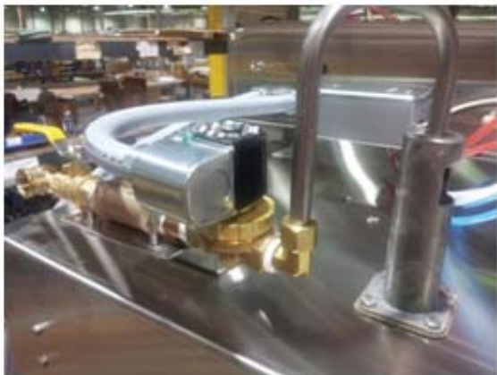
Showing 1/2" female pipe inlet, ball valve, y-line filter, water solenoid, ASSE approved air gap (backflow preventer)
