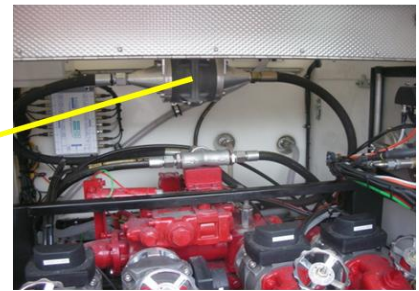
HOSE REEL(H.P.) FLOW SENSOR. (PUMP BAY REAR PANEL REMOVED TO SHOW LOCATION).
