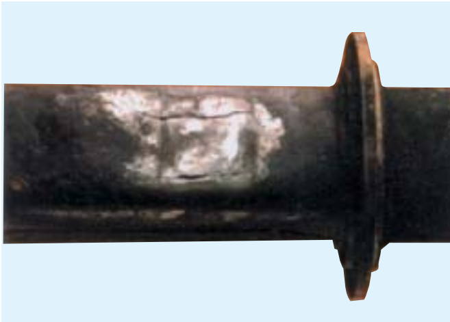
Loose Clamping Hardware
