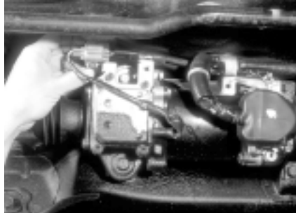
P13-2 Raise the vehicle on a lift, and check all electrical connectors on the front steering gear and rear steering actuator.
