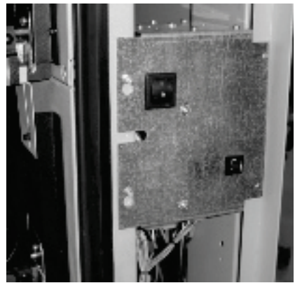
Figure 4h. Power Panel
