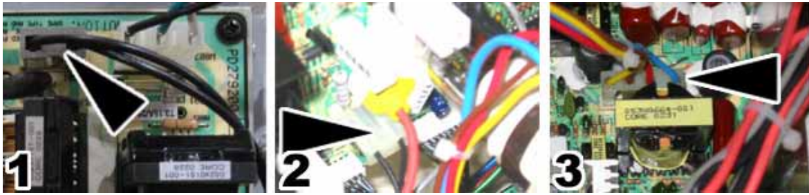
Figure 28. Monitor PCB Cables
