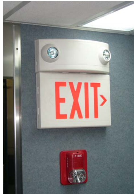
Command Area Emergency Light
