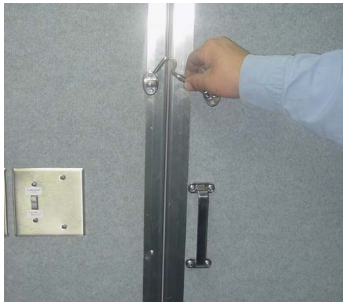
Figure 24: Secure Equipment Room Door
