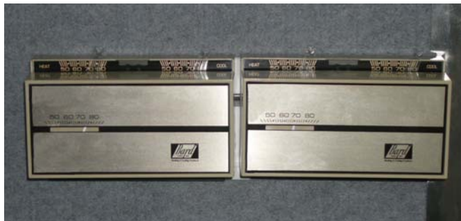
Figure 12: Mobile Unit Controls
