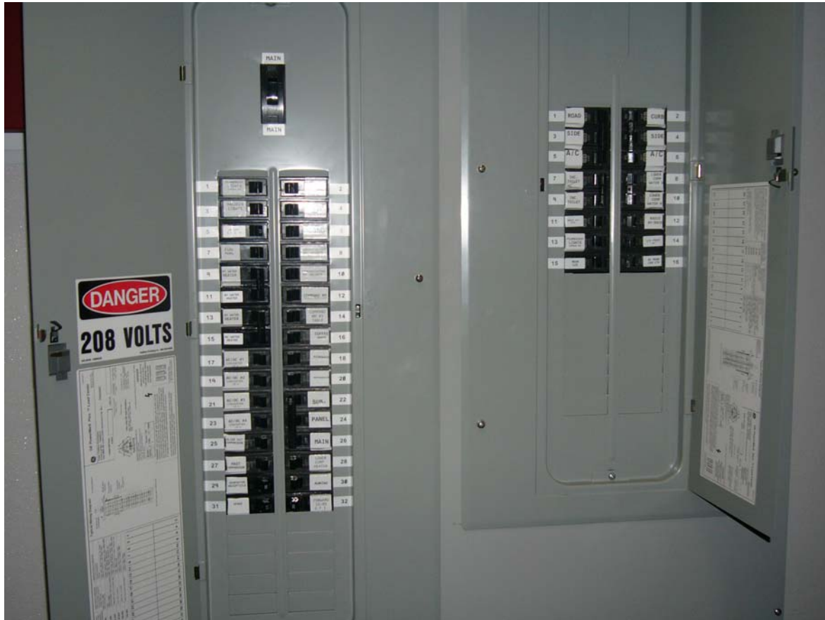
120/208V AC Electrical Panel
