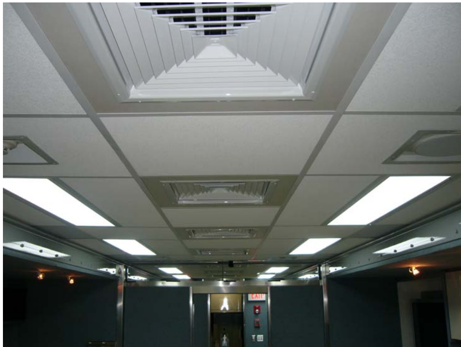
Figure 38: Command Area Overall Lighting
