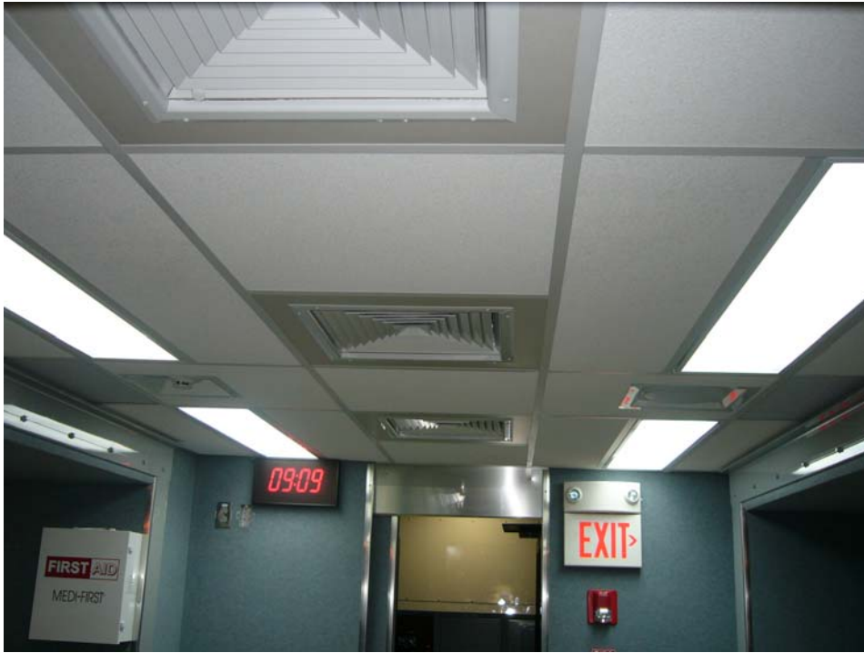
Figure 39: Communications Area Overall Lighting
