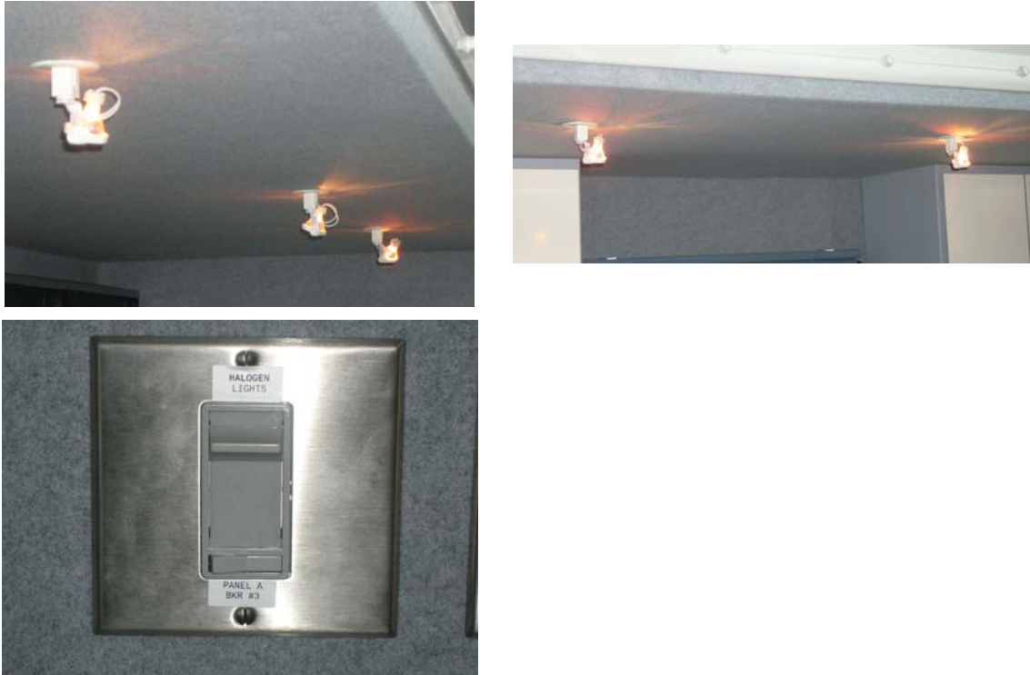
Figure 41: 24V DC Halogen Back-up Lighting & Controls
