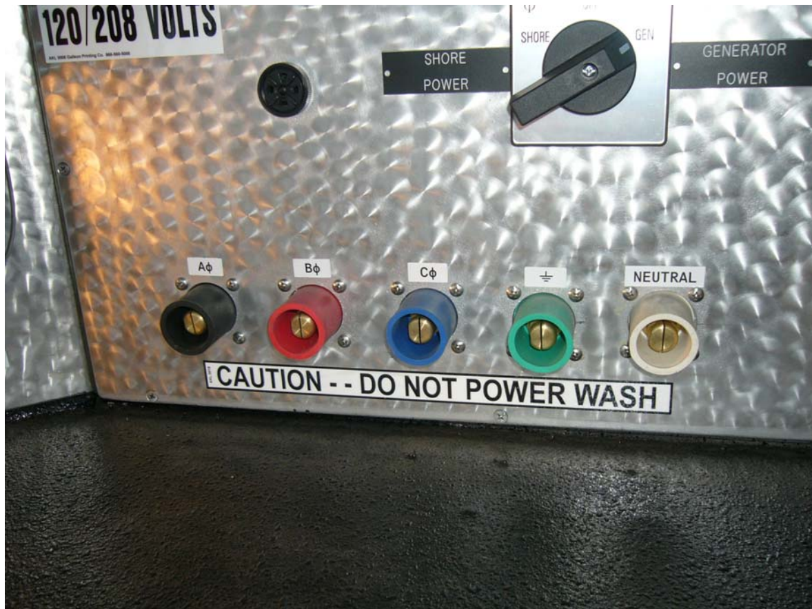
Trailer Underbody Power Connections
