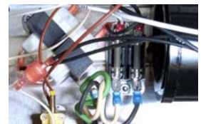
Transformer and fuses.
