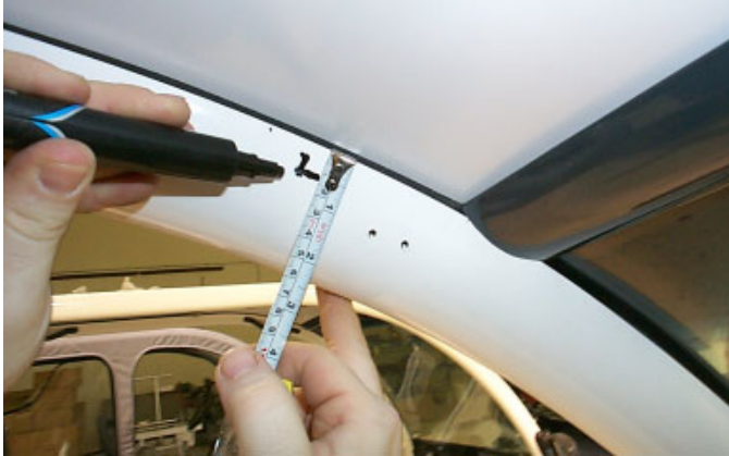
Fig. # 10 Mark and drill Ø3/8" hole in roof rail 1/2" down from ceiling
