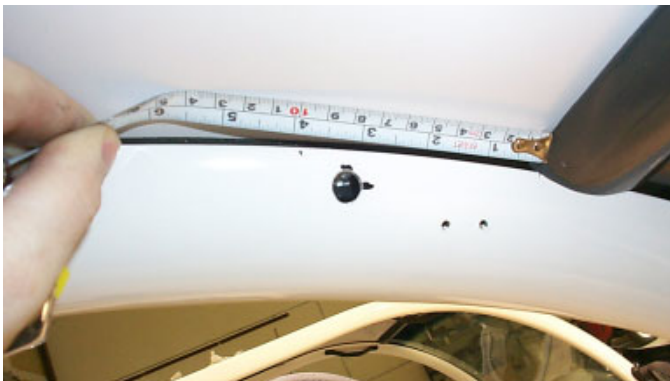
Fig. # 11 and 3-1/4" from front window brace
