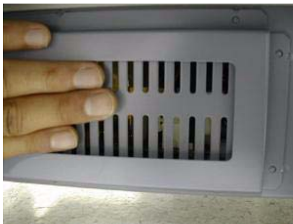
Figure 4-48 Checking Transbox fan rotating
