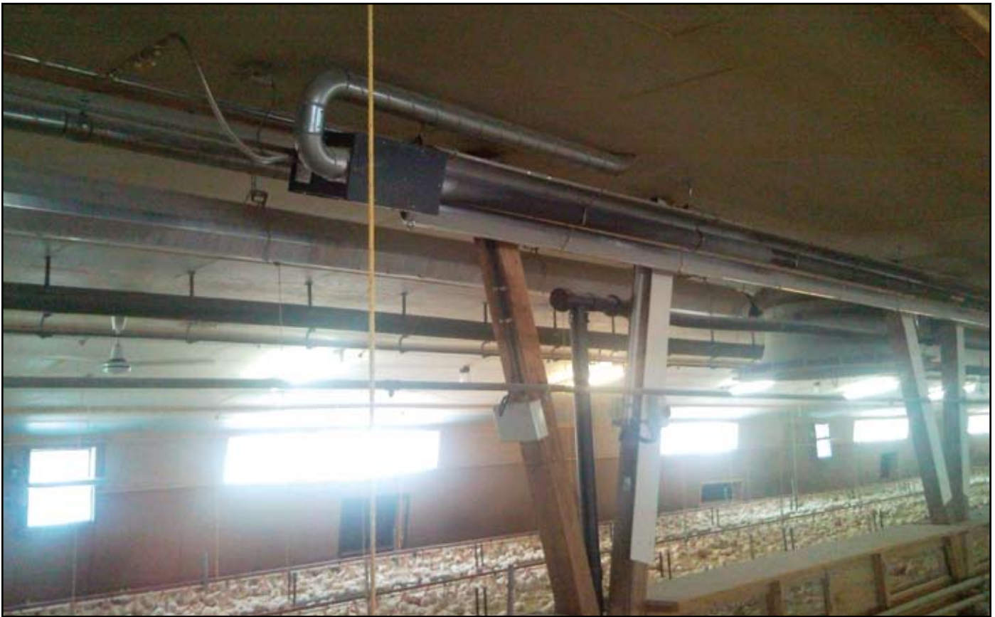
Gas-Fired, Low-Intensity infrared heaters heating a poultry house in Europe.
