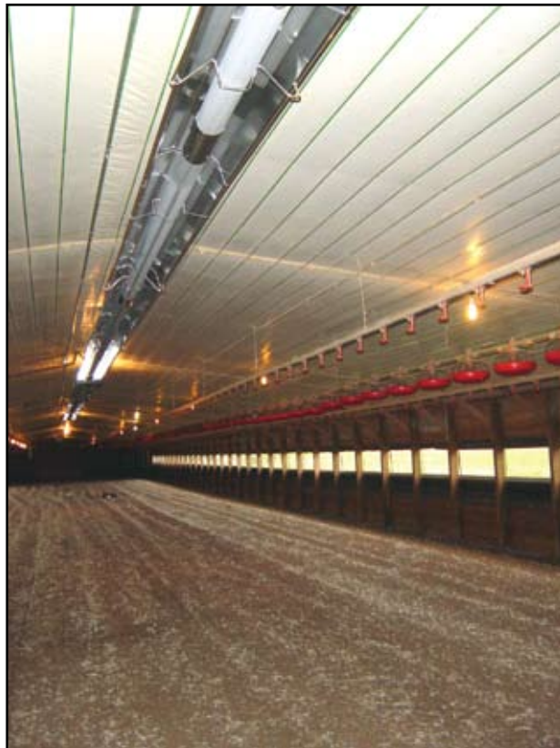
Gas-fired, low-intensity, infrared heaters are overhead and out of the way for house cleaning.
