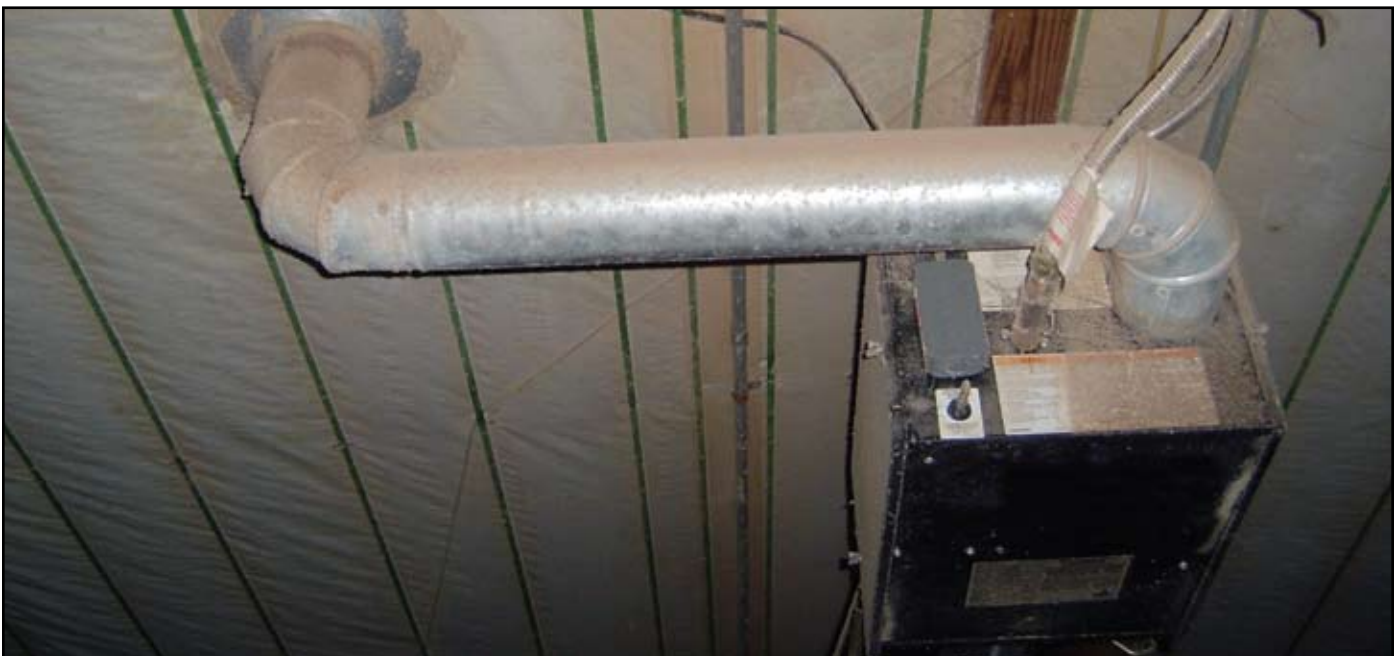
Fresh Air Intake
