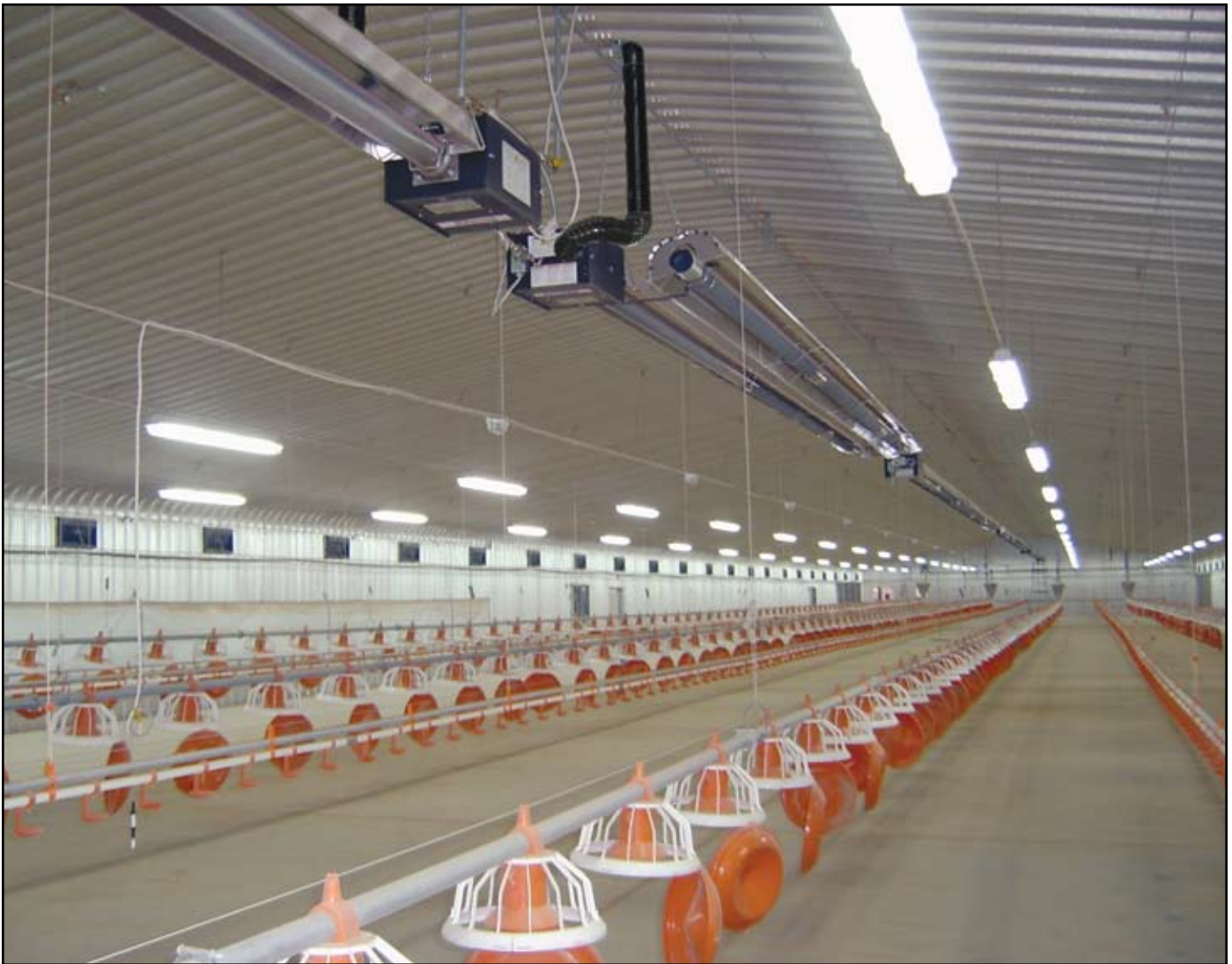
Straight and U-tube gas-fired, low-intensity infrared heaters in the same building.
