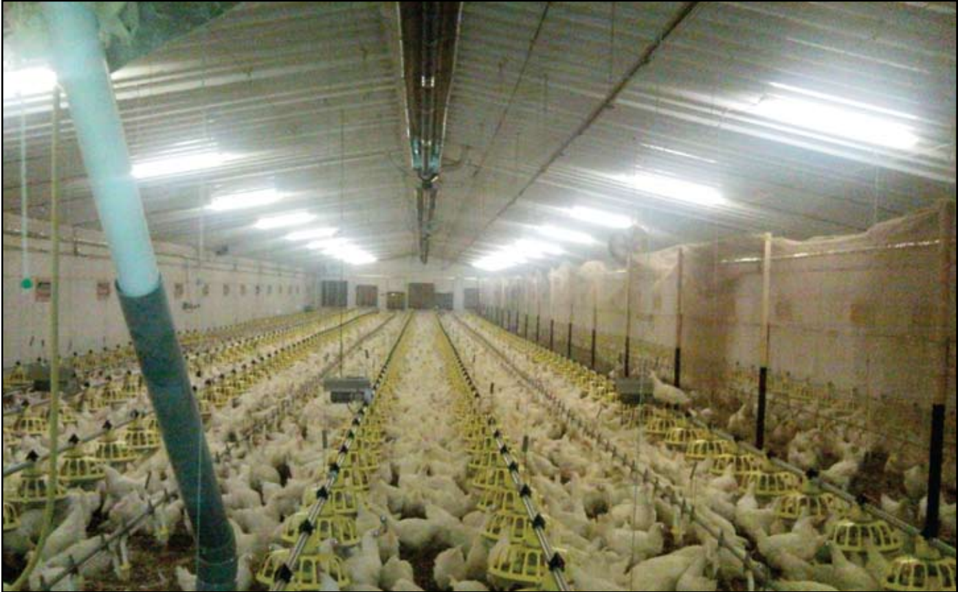
Gas-Fired, Low-Intensity infrared heaters heating a poultry house in Africa.
