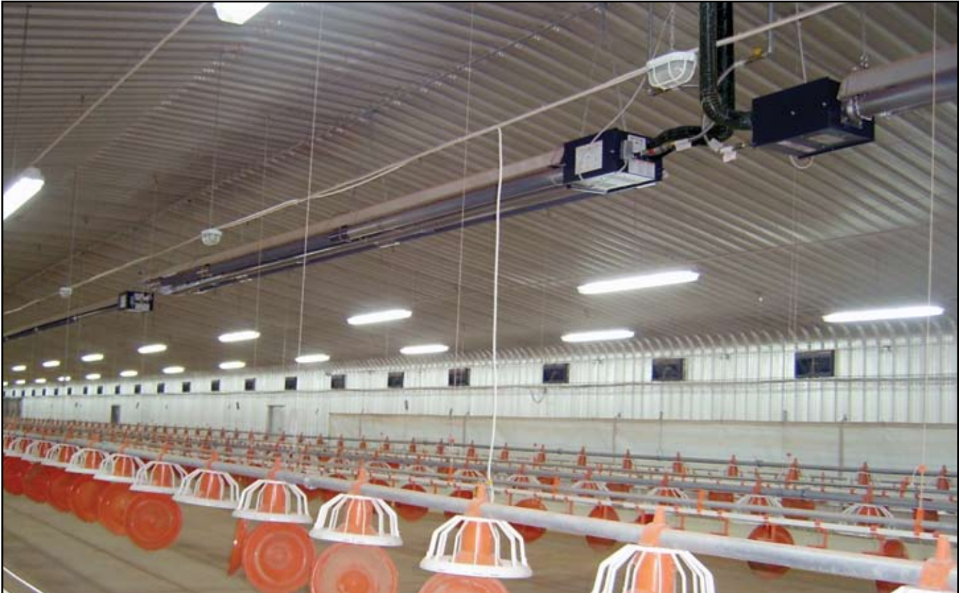
Gas-Fired, Low-Intensity infrared heaters heating a poultry house in the Middle East.
