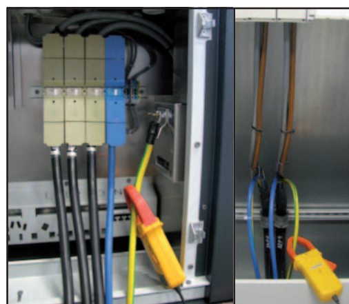
Example: Ground conductor current through ground conductor measured directly on the inverter (left) or in the distributor (right)
