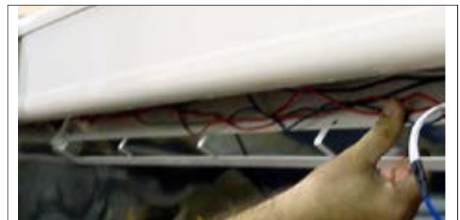
Access to Canopy and Shelf Ballasts
